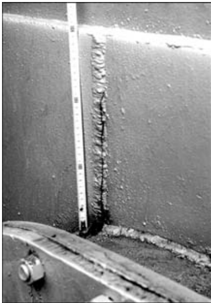
Figure 2. Crack propagation in the circumferential weld made on reinforcing coverplate of the oval hatch in the oil tank of 20,000 m 3 capacity from 09G2S-12 steel with 16 mm wall thickness
