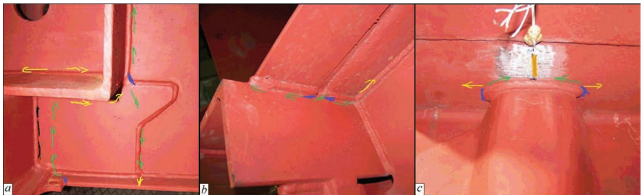
Figure 6. Crack propagation: a — in bolster assembly; b, c — in side wall rack sealing assembly
