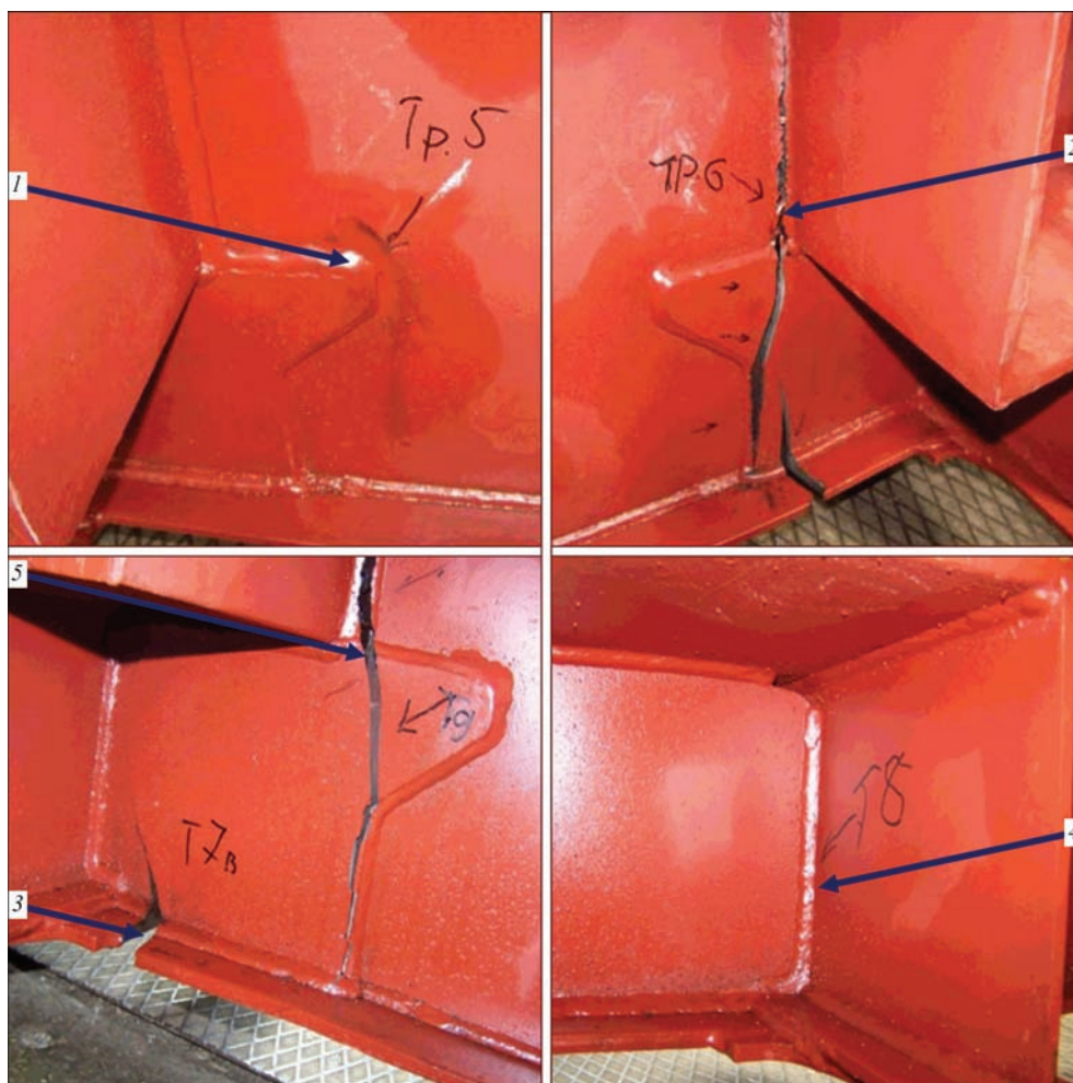
Figure 4. Cracks in bolster assembly (sample No.4): 1 — crack T5; 2 — T6; 3 — T7; 4 — T8; 5 — T9 from crack T6 on the other side from center sill
