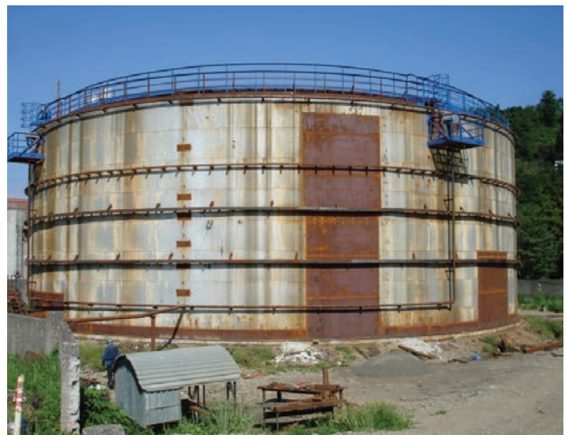
Tank with volume V = 10000 \text{ m}^3 ( D = 34.2 \text{ m} , H = 12.0 \text{ m} ) for oil storage after repair
