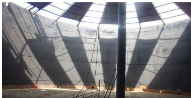
Repair of riveted tank with volume V = 5000 \text{ m}^3 built in 1895 year
