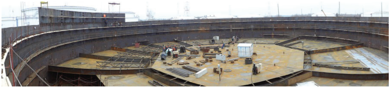
Tank with volume V = 50000 \text{ m}^3 ( D = 60.7 \text{ m} , H = 20.0 \text{ m} ) with double shell: erection the double deck steel floating roof
