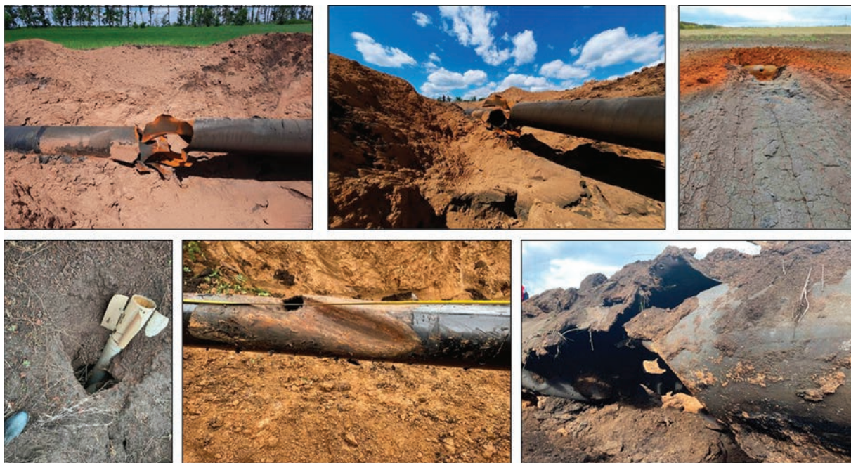
Figure 1. Pipelines damaged as a result of military operations
