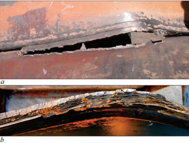
Figure 9. Fracture surface of an X70 steel pipeline in the vicinity of a corrosion crack formed during service of a 1420×15.7 mm TP
