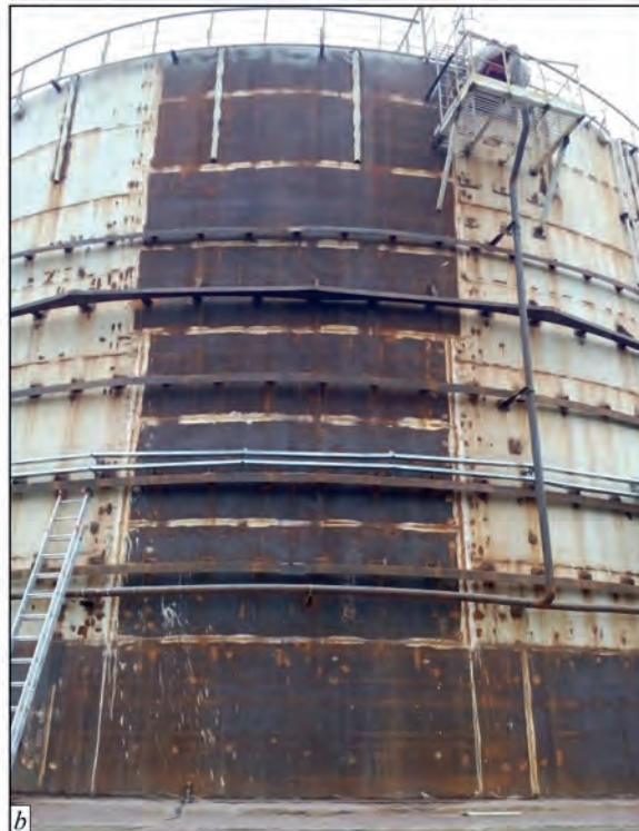
Fig. 1. Process of tank repair: a – design schema; b – shell after installation stiffening rings, tank is empty
