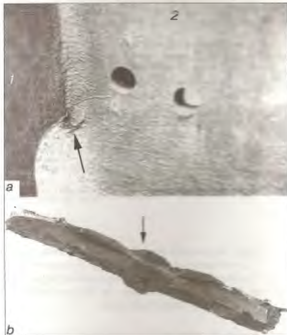
Figure 3. Lamellar-fatigue fracture of a bridge framework: a — fracture site (1 — stiffener; 2 — load-carrying beam); b — fracture site on a fragment (shown by an arrow)
