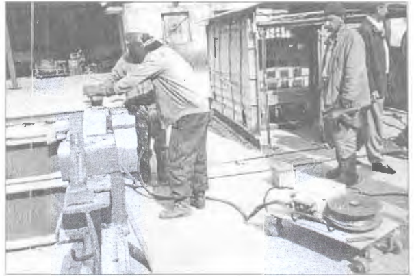
Figure 4. Use of PSh-107R semi-automatic machine for cutting out a technological hole in an electrolyzer case
