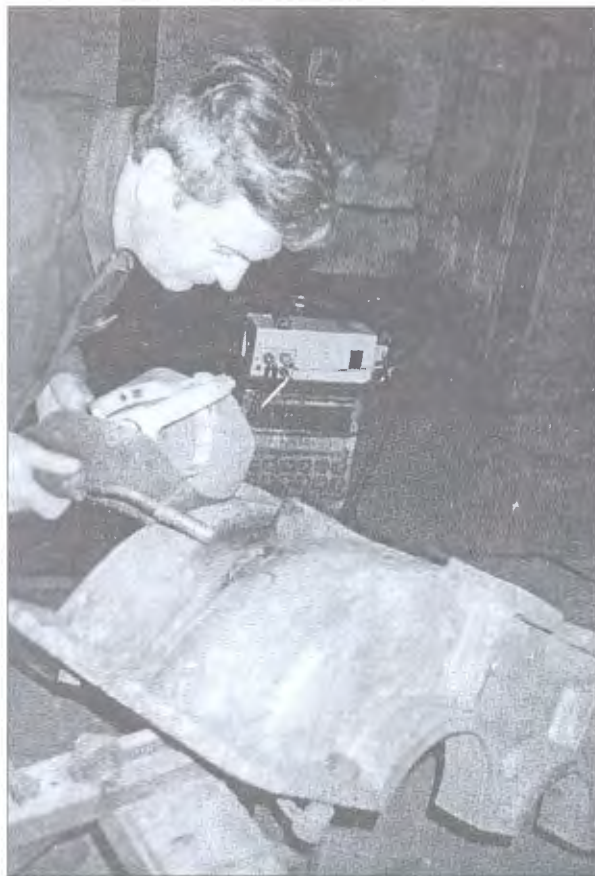
Figure 8. Welding up a crack in the case of a reduction gear using PSh-107G semi-automatic machine
