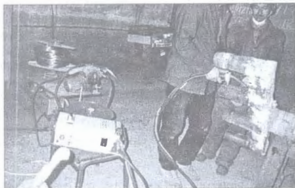
Figure 2. Welding of a boss to anode-holder (circumferential welds) with PSh-107V semi-automatic machine
