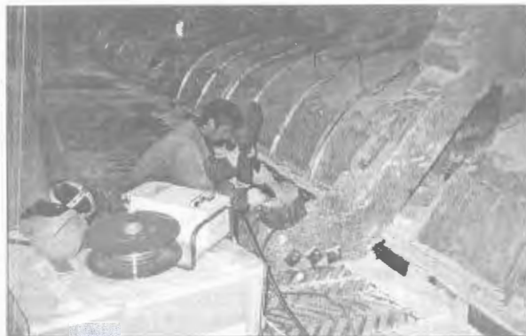
Figure 10. Repair welding of elements of an aluminium busbar in an operating electrolyzer with semi-automatic machine PSh-107VA using magnetic shields
