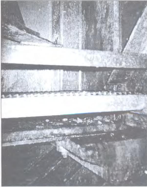
Figure 2. Appearance of corrosion damage of booms, ribs of main beams, joint members in over-supporting members of framework in the E.O. Paton bridge
