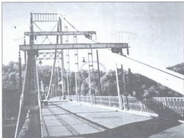
Figure 5. The Park pedestrian bridge to Trukhanov island with devices for unloading of suspension rods
