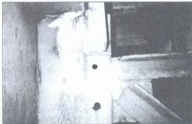
Figure 7. Appearance of longitudinal crack in side fillet weld of fastening of suspension rod to vertical rib on the main beam wall of the Park pedestrian bridge to Trukhanov island
