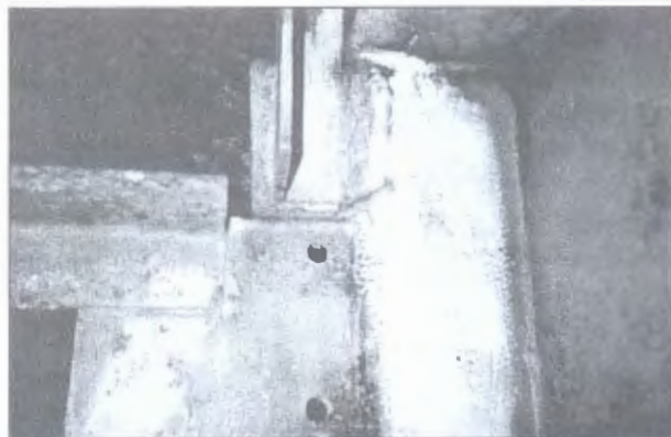
Figure 6. Appearance of fatigue crack in unit of suspension rod fastening in the Park pedestrian bridge to Trukhanov island where a distance between side and end fillet welds is not observed
