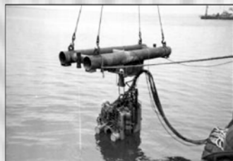
Lowering under the water of the flash-butt welding machine used for welding pipelines
