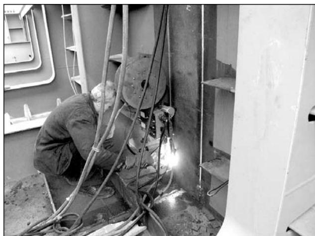
Figure 5. PP-AN9N flux-cored wire welding with forced formation of vertical butt joints on snap structures of Podolsko-Voskresensky Bridge over the Dnieper River in Kiev
