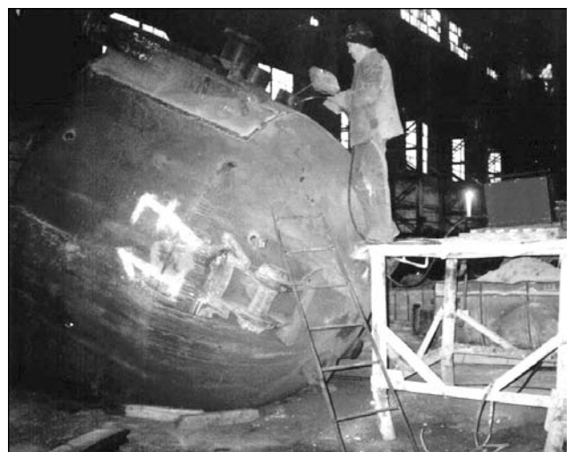
Figure 4. Repair welding of metallurgical equipment with flux-cored wire PP-AN7 at OJSC «F. Dzerzhinsky Dneprovsky Metallurgical Works, Dneprodzerzhinsk [5]
