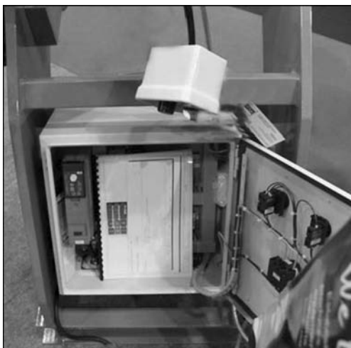
Figure 3. Control unit of valve electric motor
