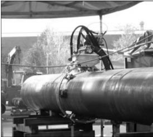
Figure 8. Entire test set-up on the pipe
