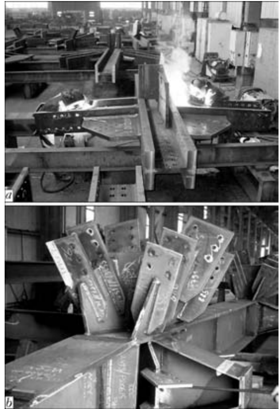
Figure 8. Pre-production of the gusset plates for «Eurasia» (a) and «Shakhtar» (b) using flux-cored GMAW in Gemlik
