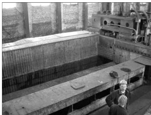
Figure 9. Shearing machine hopper lined with plates after plasma hardening
