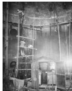
Completion of repair of blast furnace (inside view) at «Krivorozhstal» Works. As-welded part of wall is shown
