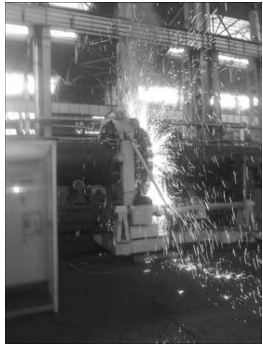
Figure 16. Complex for flash-butt welding of offshore pipelines of 1219 mm diameter and 27 mm wall thickness
