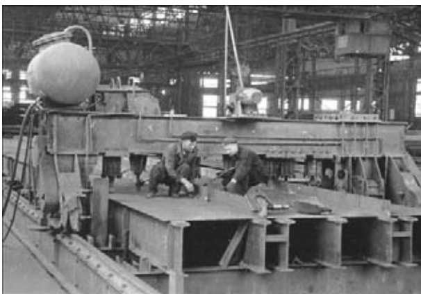
Figure 2. General view of the rig cross-arm for assembly and welding of large-size assembly elements in the workshop of plant of metal structures in Dnepropetrovsk
