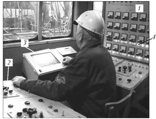
Figure 3. Central cabin of control of installation machines: 1, 2 – respectively, control panels of right and left blocks; 3 – industrial computer PC 670 of system of welding conditions monitoring; 4 – signal lamps of control of welding wires movement
