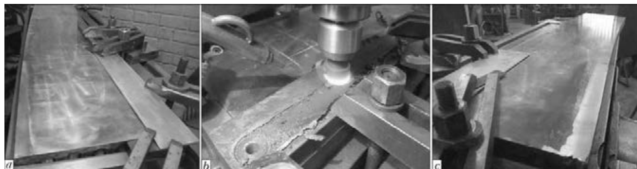
Figure 7. Stages of deposition of copper layer on copper plate: a – plate with thin copper sheet; b – surfacing process; c – appearance of restored plate after grinding
