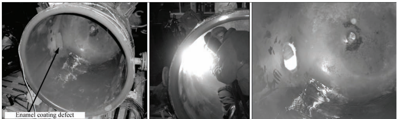
Figure 6. Process of restoration of local damages of enamel coating of V-630 reactor using microplasma spraying method under production conditions
