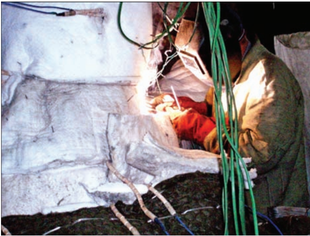
Figure 7. Performing repair welding of a crack in the body of the MCP control valve
