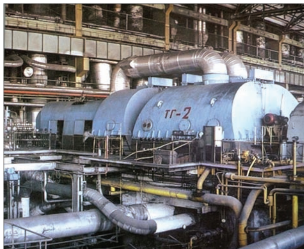
Figure 1. General appearance of turbine PT-200-130
