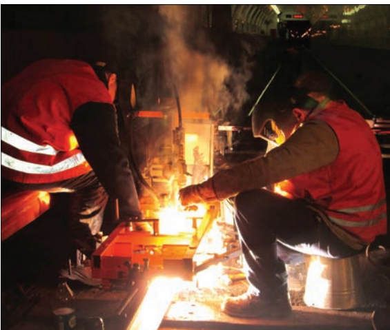
Figure 2. Automatic consumable electrode electric arc bath welding in the tunnel of Kyiv underground
