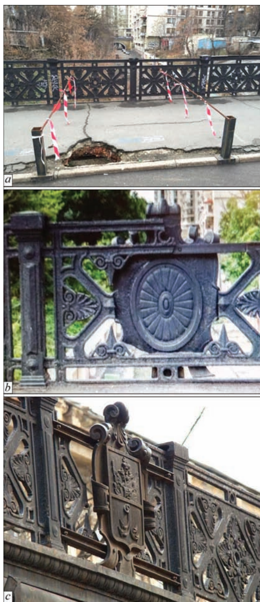
Figure 2. General view of condition of the railing of the Kotzebue bridge in 2016 (before disassembly): a — panoramic view; b — rear side of the emblem on the under emblem grate; c — front side of the emblem on under emblem grate
