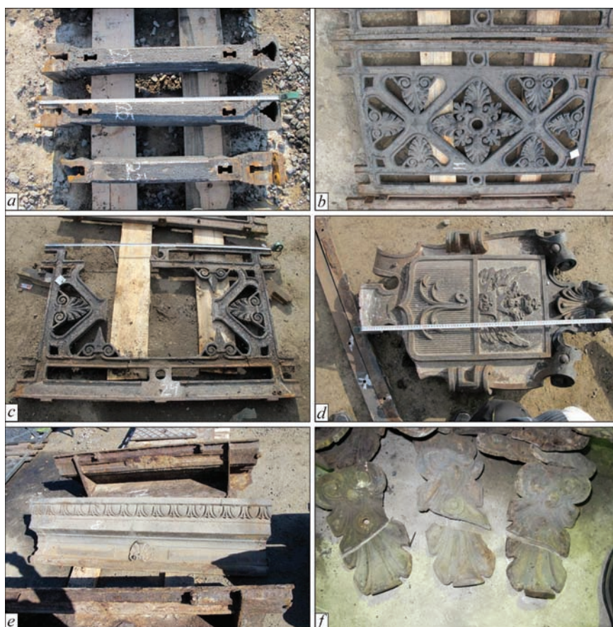
Figure 4. Examples of condition of characteristic parts of railing, established during expert examination: a — poles Nos 25, 26, 27; b — grate No. 11; c — under emblem grate No. 24; d — emblem No. 1; e — cornice No. 8; e — corner elements of decor Nos 1, 2, 3
