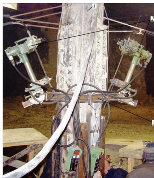
Figure 4. Fastening A-1304 machines on a building column: 1 — column; 2 — welding machines; 3 — quick-detachable frame
