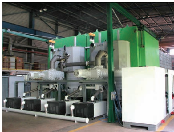
Figure 3. Electron beam installation with a vacuum chamber of 100 \text{ m}^3
