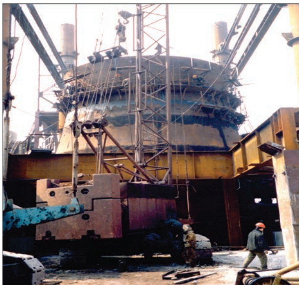
Figure 7. Repair of blast furnace DP-2 at the OJSC «Azovstal Steel Plant» using rolled steel 06G2B of the strength class C440
