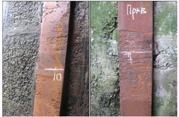
Figure 5. Characteristic damage of working path rails of lift gates in Kaniv navigation lock
