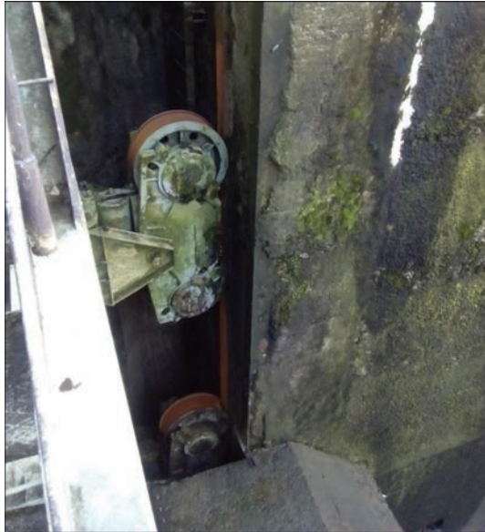
Figure 3. Support carriage of lift gates in Kaniv navigation lock work gates and penstocks is activated by volumetric hydraulic drives.
