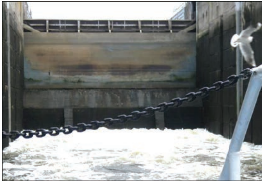
Figure 2. Lift gates of Kaniv navigation lock
