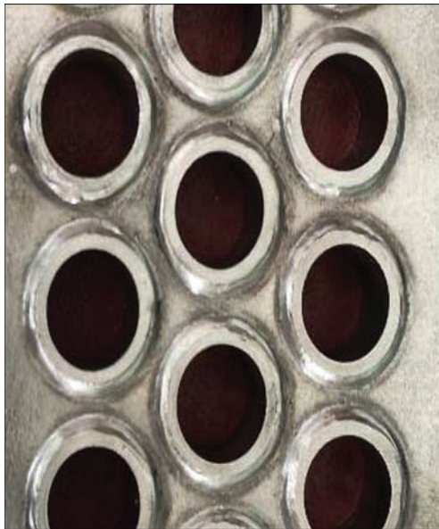
Figure 9. Appearance of welded joints on simulator-samples with plugs welded by laser process
